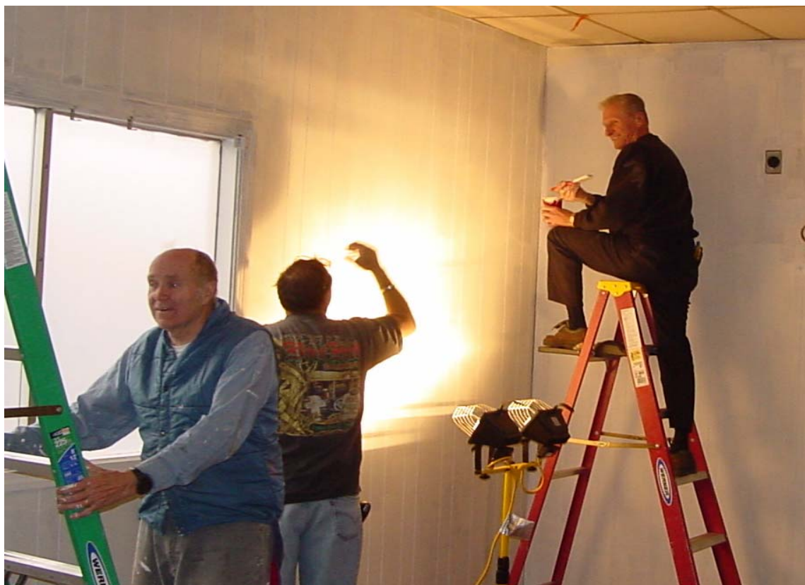
A WORK IN PROGRESS ADHERING TO THE NEW FIRE CODE REGULATIONS AT THE HALL Applying fire-retardant paint to the Hall walls are, from left to right, Frank Item, Ron Travers and John Silvia.
