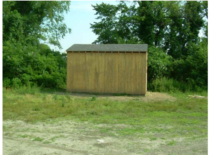
The shed is nearing completion. This photograph shows the progress of the project as of June 27, 2008
