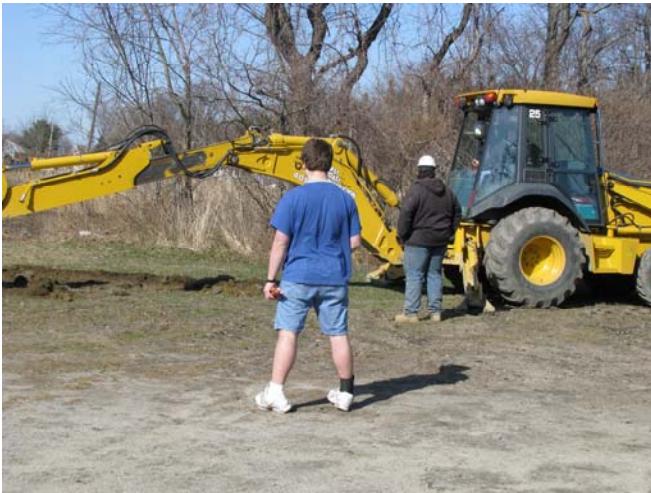
Ben tentatively watches as the process begins. East Coast Construction breaks ground where the shed will be located.
